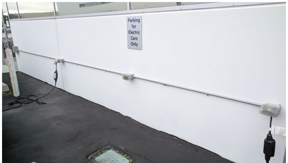
Figure 1 Multiple 120-volt outlets mounted along an external wall provide easy access to Level 1 charging. EV owners use the Level 1 cord set that is typically provided with purchase or lease of the vehicle.
