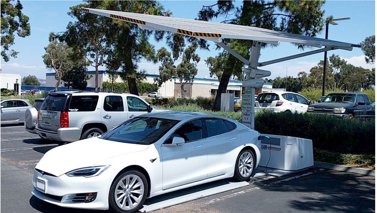
Figure 4 An EV charging under a stand-alone solar canopy. The solar photovoltaic panels charge a battery that then charges the vehicle. The solar canopy does not interconnect with the building’s electrical system.
